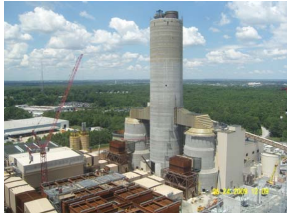
Partially completed new scrubber project chimney stack at the Brandon Shores power plant.
